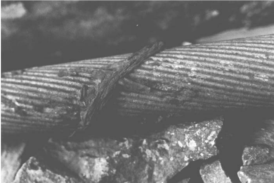
Figure 8.8 Deposit corrosion underneath remnants of jute on a 24-year-old sea cable. (Photo: Steinar Refsnæs, EFI, Trondheim.)
