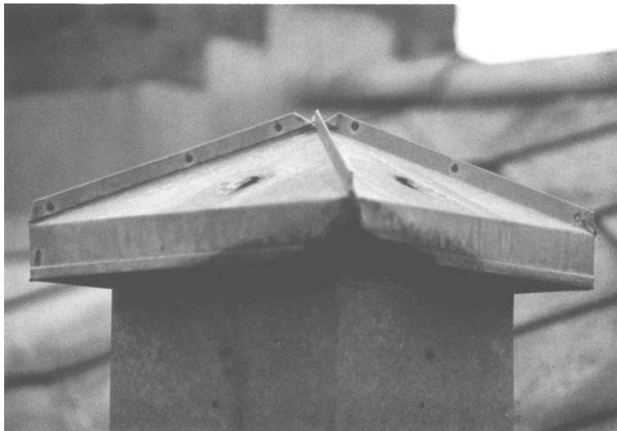
Figure 8.1 Corrosion damage of a 14-year-old ventilation outlet from a bathroom in a private house. (Photo: Sigmund Bardal.)
